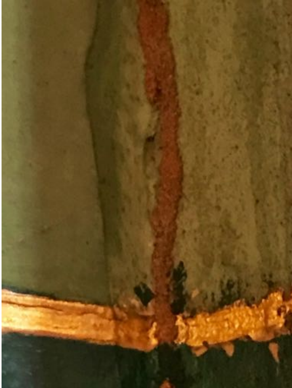
Termites have formed a tunnel in the plaster-on-wood wall of this monastery Lhakhang. The wall painting is disturbed, and the termites are causing structural damage to the building.
