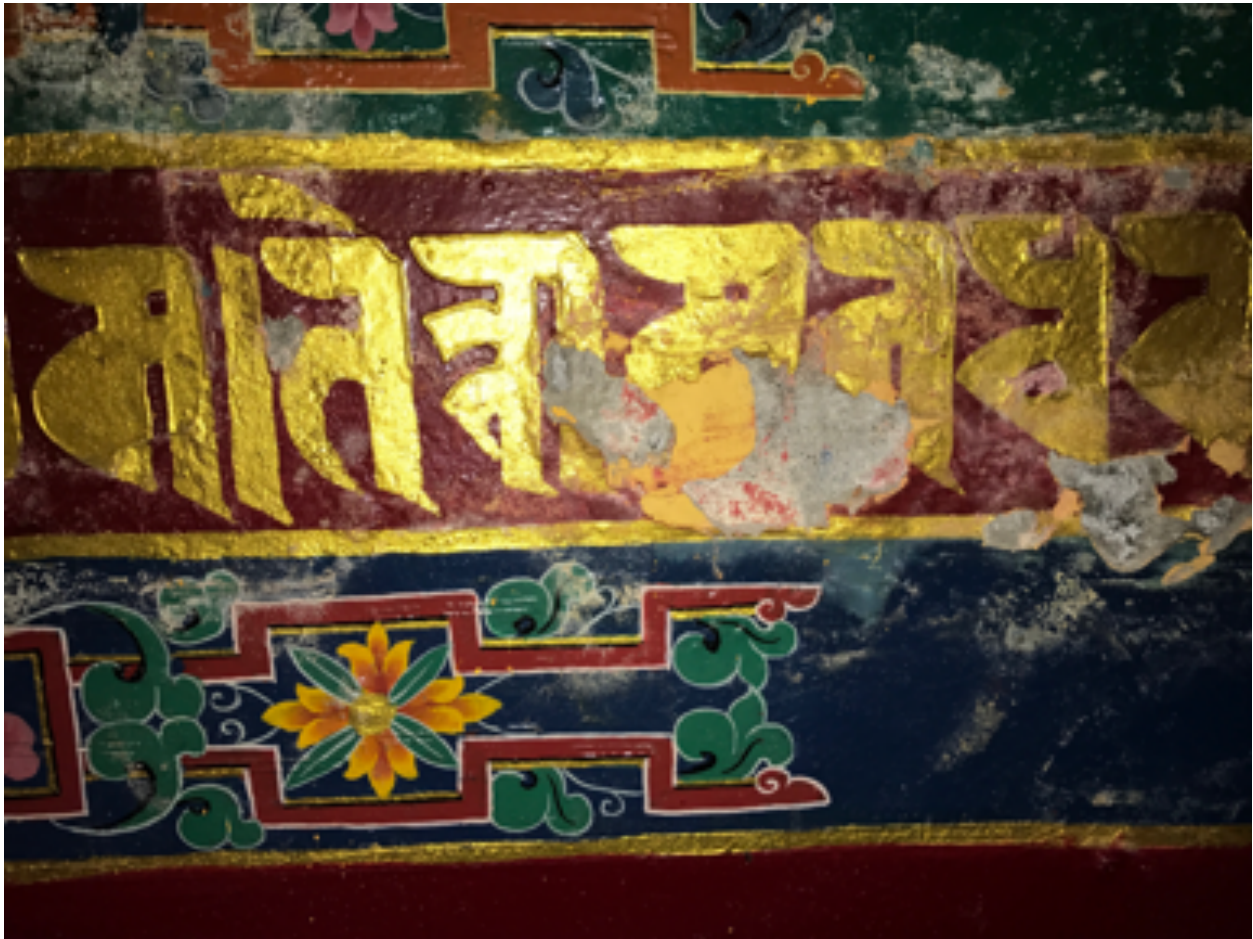
This wall painting became damaged by water. You can see the raw concrete beneath where the paint has flaked away.
