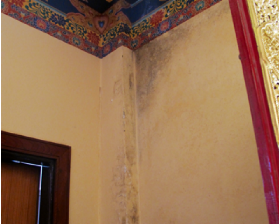
There was a roof leak up at the top and this caused mold. This is what happens when water comes through the walls.
