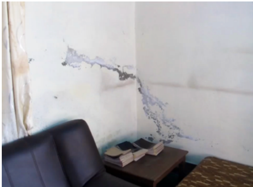
In this monastery office, dampness is rising through the concrete wall due to the damp ground outside of the building and due to earthquake damage to the building
